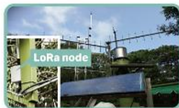
水文站監測傳輸 Hydrological station monitoring transmission
